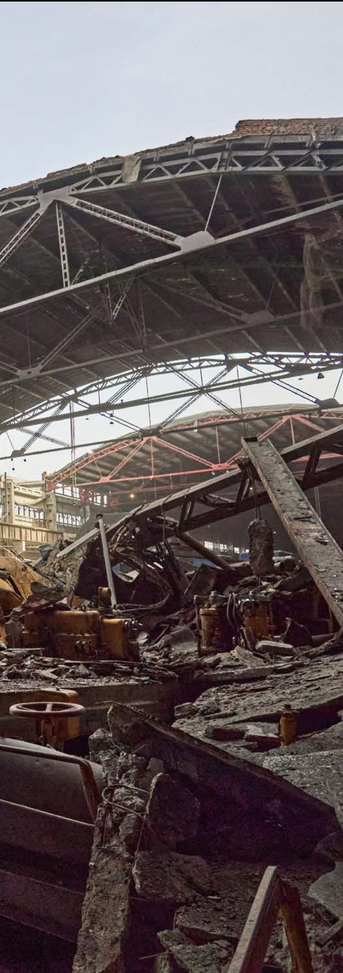
Power unit machinist Dmytro surveys the remains of a once-bustling control room. Serge Serdiukov, 2024
