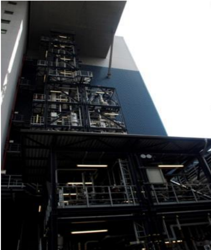
CCS demonstration project, Niederaußem power station (RWE), Germany, photo taken in Sept 2011
